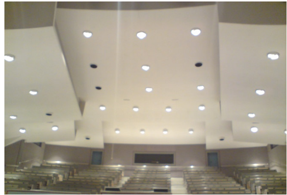
Figure 6. Suspended ceiling of Hebb Theatre Source: Photo taken by Kristen Ferma - March 2, 2010
